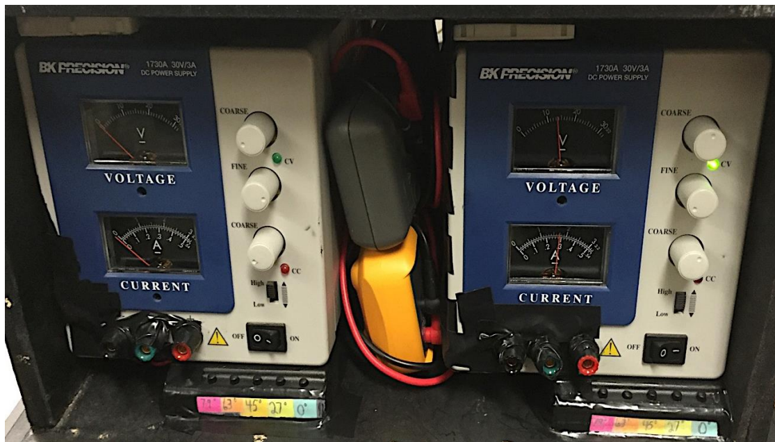
Figure 32. Upper Level Power Control Section
